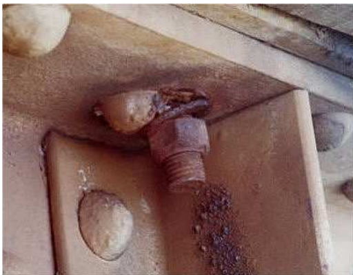
Traditional method of attaching ties to bridge deck. Repairs are needed weekly to retighten loosened bolts
